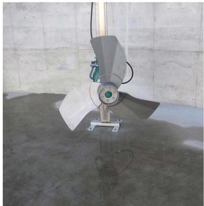
4G with EV - Open tank
